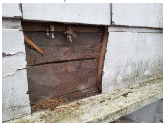
Picture 5. Wooden materials in bad shape
