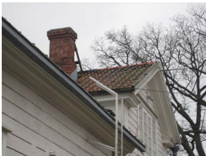
Picture 8. Bad covering materials
