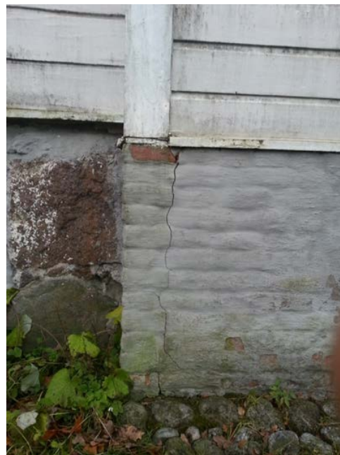
Picture 2. Settlement cracks
