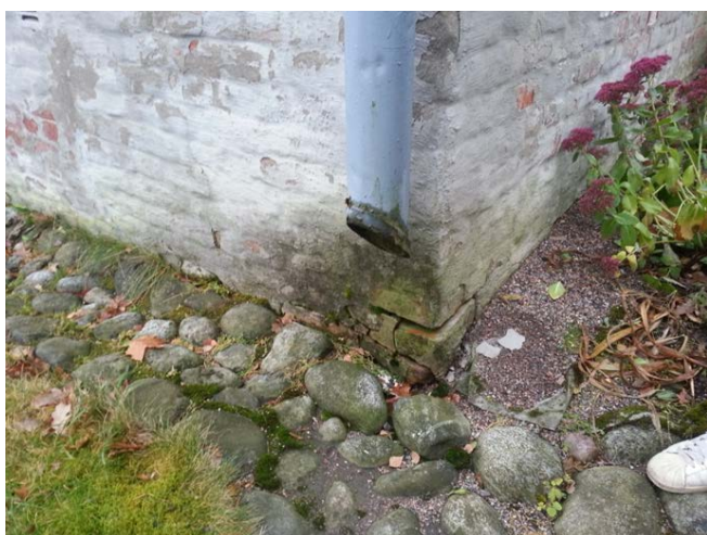
Picture 3. Water damage
